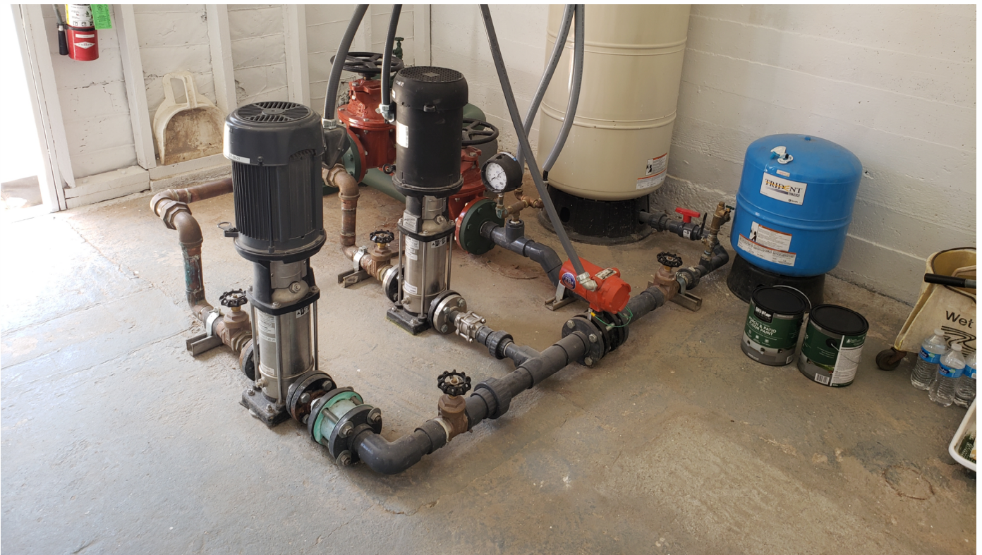
Figure 2-10. Hierba Pump Station
