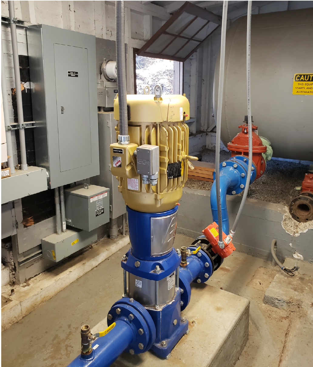
Figure 2-11. Alegre Booster Pump Station
