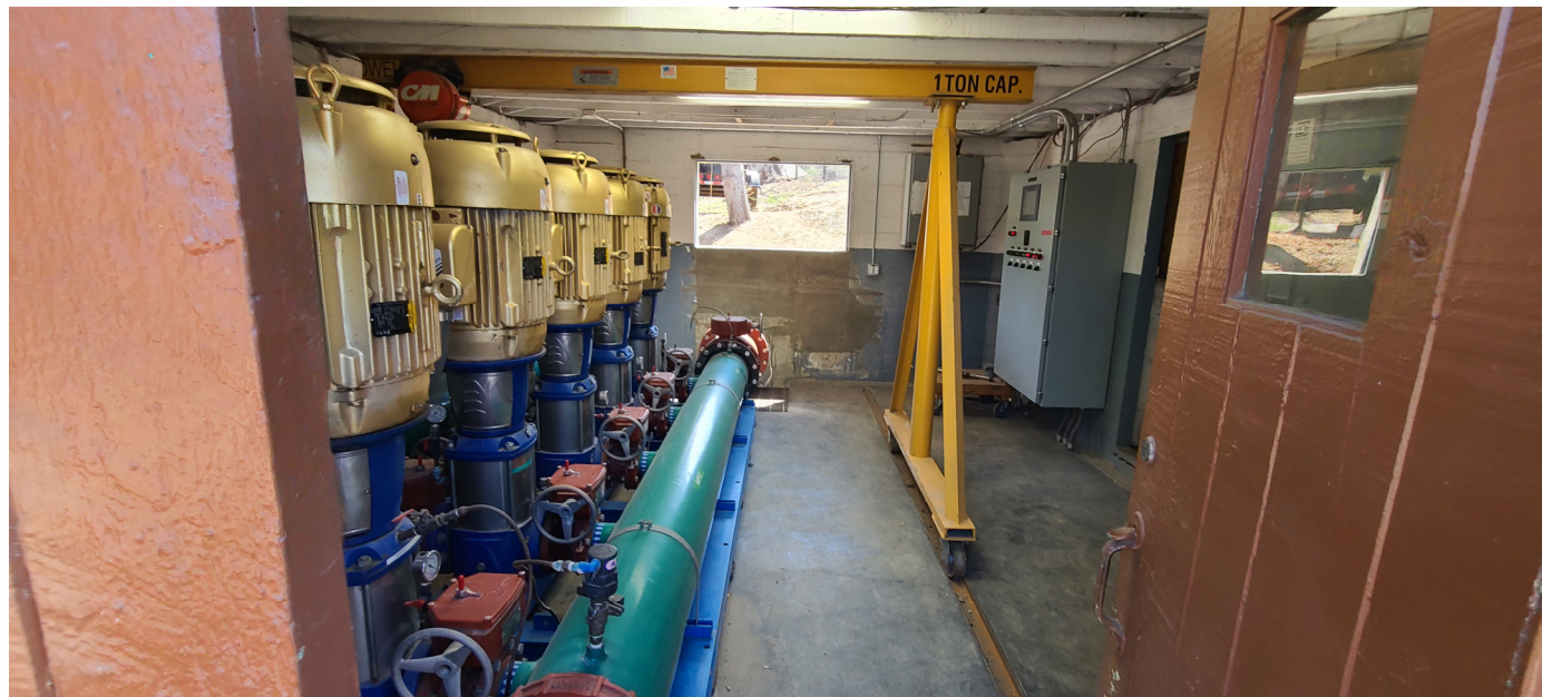
Figure 2-7. Tranquila Booster Pump Station
