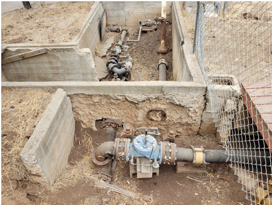
Figure 6-1. Modoc Pressure Relief Valve
