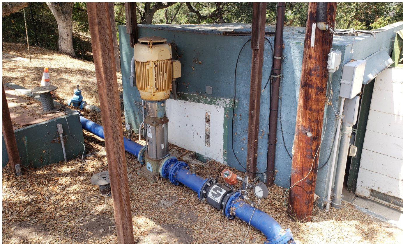
Figure 2-8. Cresta Booster Pump Station
